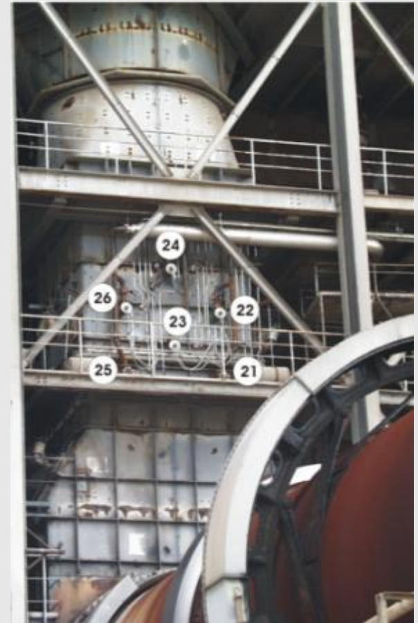
Injector configuration in the riser duct of a rotary cement kiln
